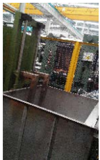
Water cooling device
